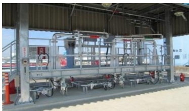
Drum filling facilities
