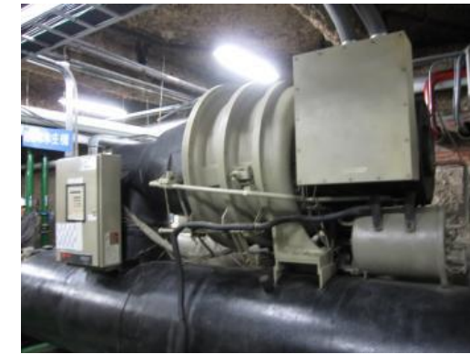
VFD Centrifugal Chiller
