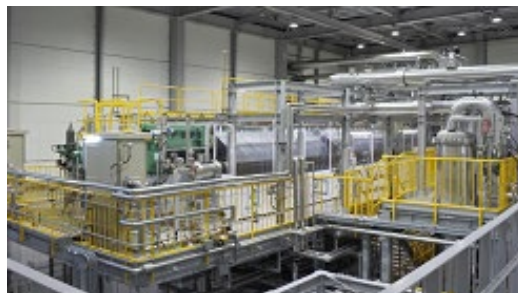
Hydrogen Production through Water Electrolysis Using Power from Renewables
