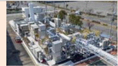
Hydrogen power generation facility (hydrogen CGS) constructed on Port Island in Kobe City
