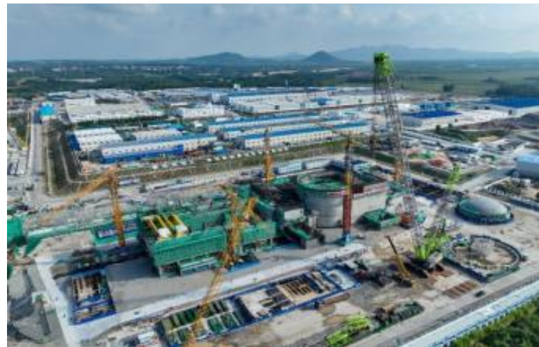
ACP100 unit in Hainan Province
