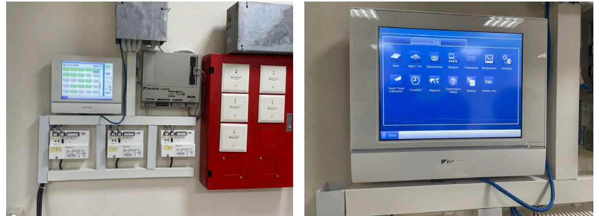
HVAC Automation System
