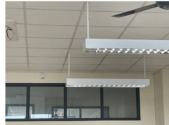
Lighting Automation System
