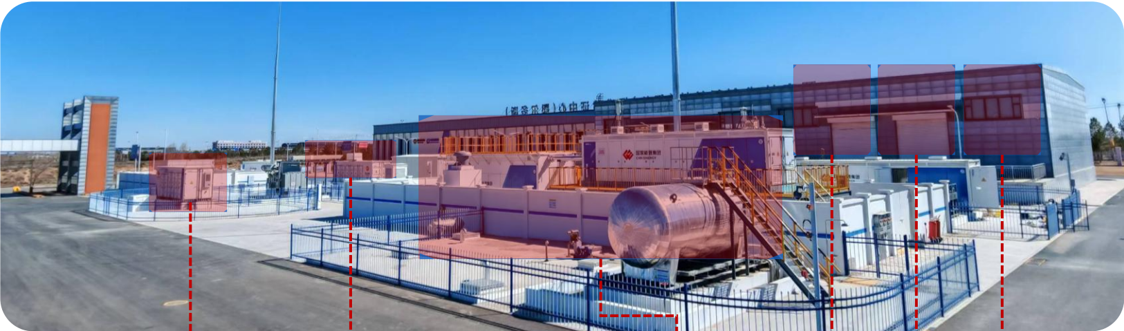
No. 1 Test Site of the Industrial-Scale Green Hydrogen Equipment Testing and Validation Research Center
