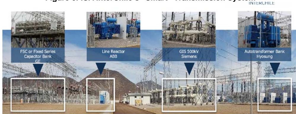
Figure 6: ISA InterChile’s “Smart” Transmission System
